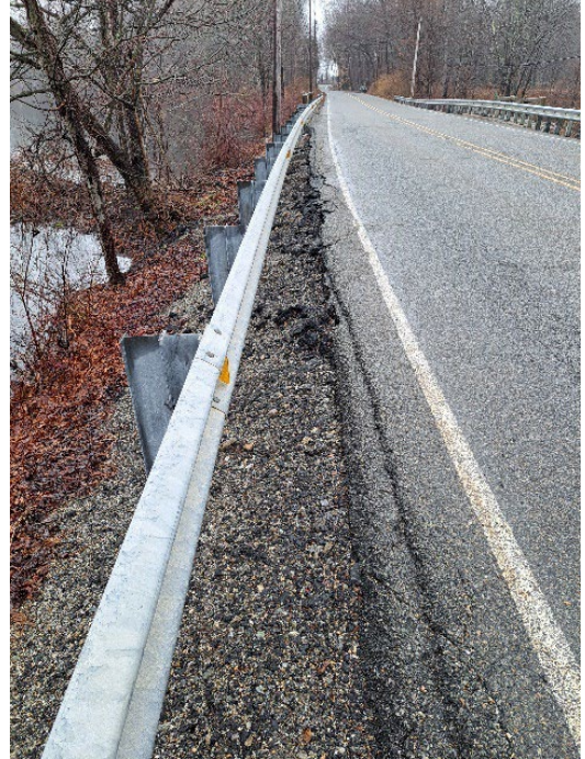
Photo 8-27: Shows edge of road degrading from surface runoff and gravel washout (Recommendation 11A)
