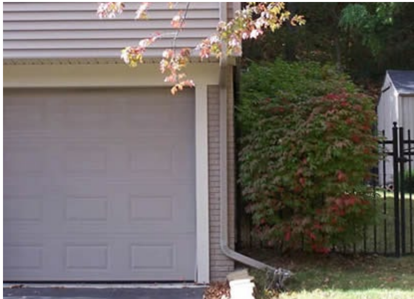
Photo 9.2: Downspout Disconnection, Source: USEPA
