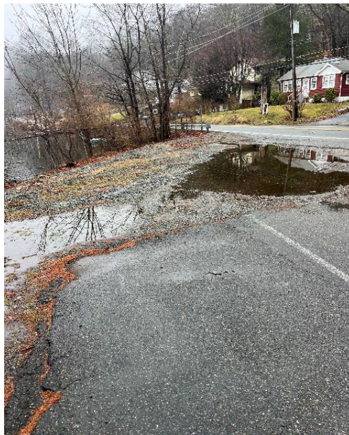
Photo 8-3115: The south end of the parking lot with excess road gravel and pooled water (Recommendation 12B)
