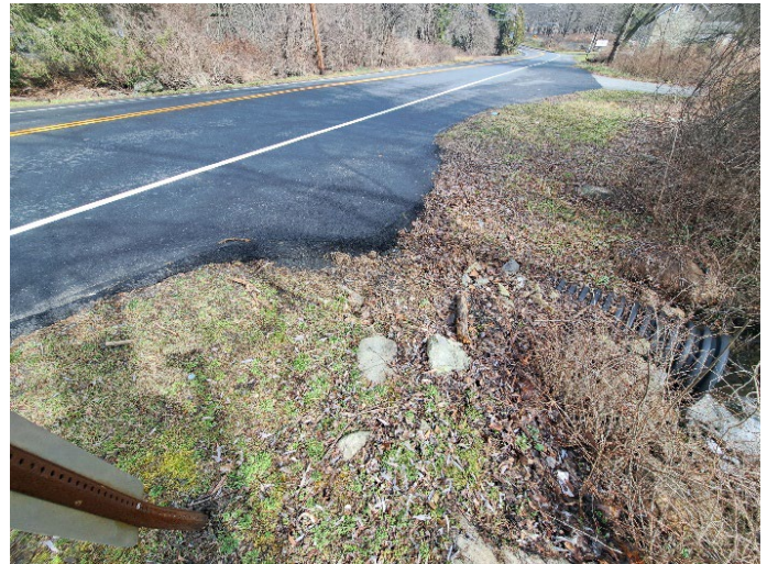
Photo 8-20: Misaligned channel and bank erosion along culvert headwall (Recommendation 7B)
