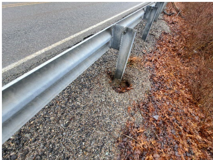
Photo 8-28: Scour hole is being formed along the guardrail support from stormwater runoff (Recommendation 11A)
