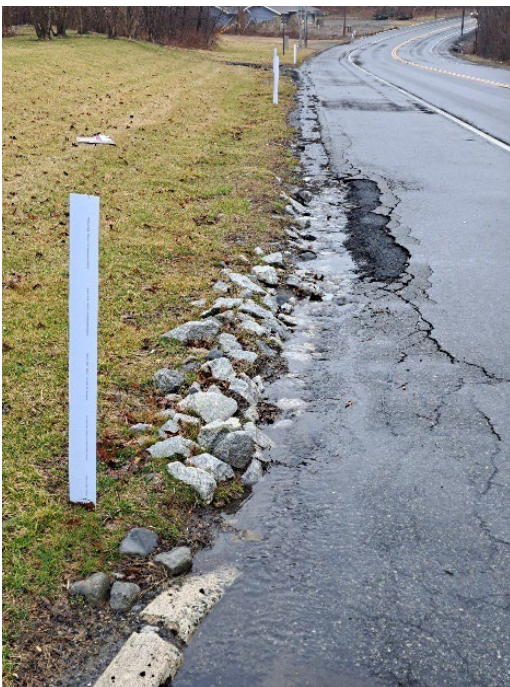
Photo 8-49: Stormwater Runoff along Rt 206 North in front of Metro Self Storage (Recommendation 21A)
