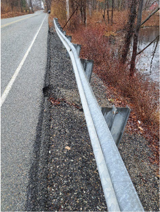
Photo 8-26: Erosion forming along the Roseville road base (Recommendation 11A)
