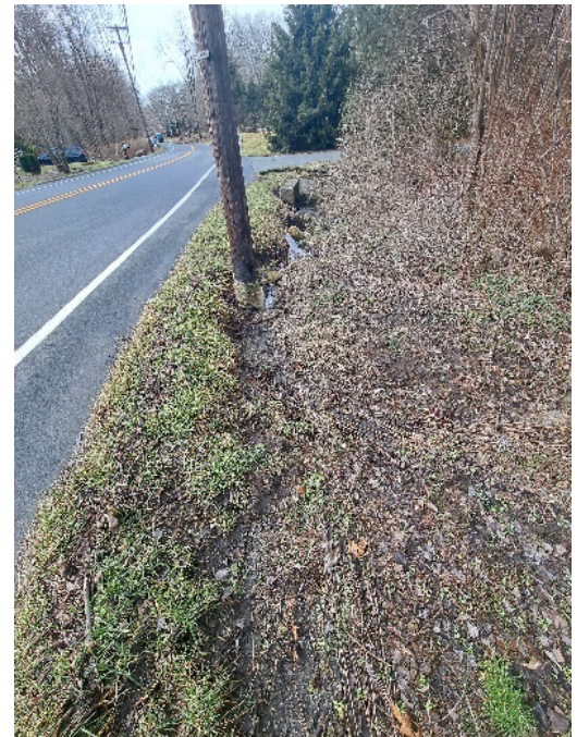
Photo 8-148: Active erosion around utility pole from stormwater runoff (Recommendation 7B)
