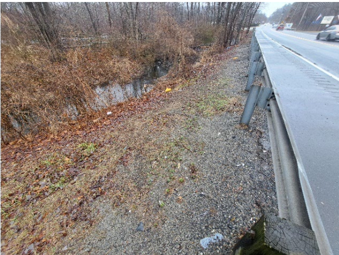
Photo 8-42: Gravel bank by guardrail along 206 (Recommendation 18B)
