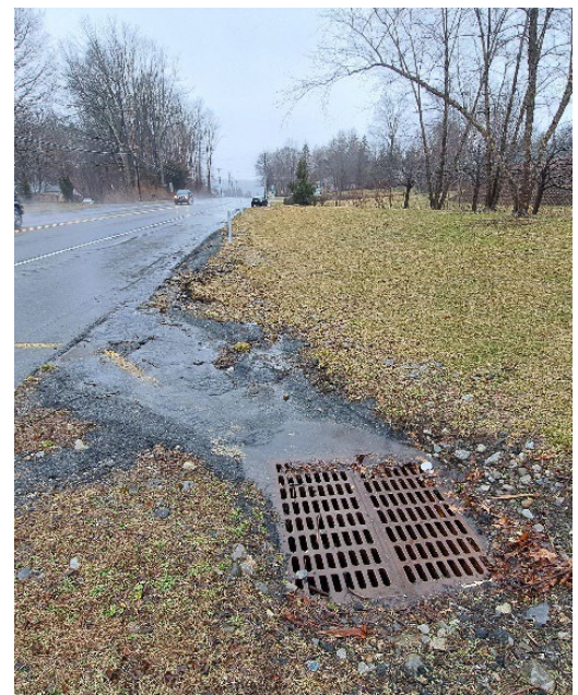
Photo 8-50: Stormwater Runoff along Rt 206 North in front of Metro Self Storage (Recommendation 21A)
