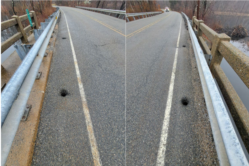
Photo 8-29: Holes to drain road runoff directly into Wolf Lake (Recommendation 11B)
