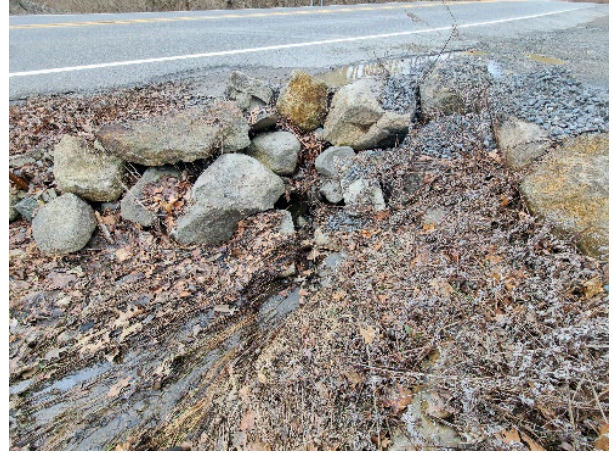
Photo 8-22: The culvert is being partially blocked by the riprap and is becoming clogged with driveway material and plant matter (Recommendation 8A)
