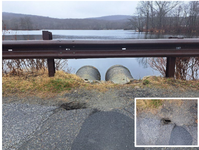
Photo 8-53: View of the overflow culverts looking toward Jefferson Lake. The inset is an overhead view of the hole in the road deck that drains into the culvert on the left (Recommendation 22C)
