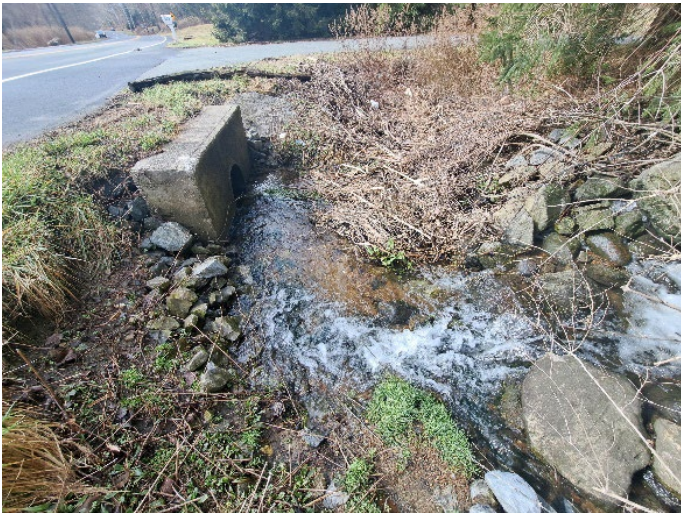
Photo 8-19: Downstream section of culvert showing exposed HDPE pipe and potential for erosion along edge of the road (Recommendation 7B)
