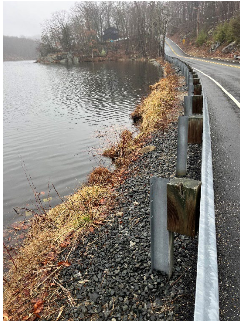
Photo 8-25: The shoreline of Johnson Lake along Tamarack Rd (Recommendation 10A)
