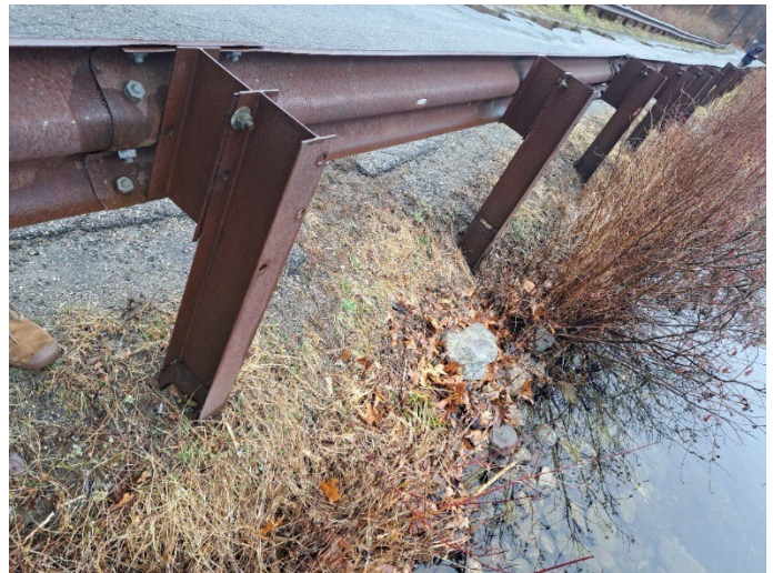
Photo 8-52: Shore erosion around rusting guardrail posts (Recommendation 22B)
