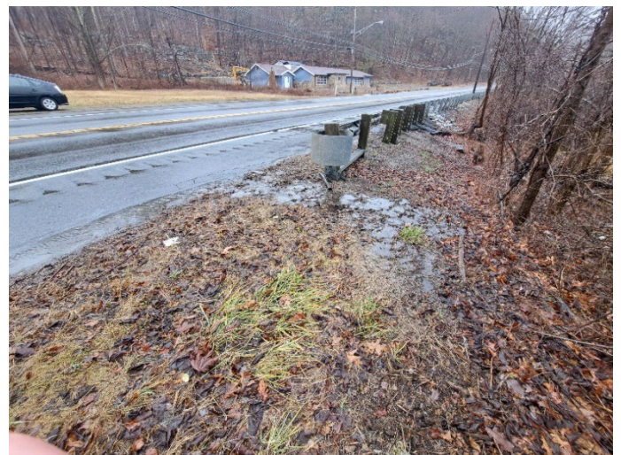
Photo 8-48: Storm runoff rills in front of guardrail toward wetland complex (Recommendation 20B)
