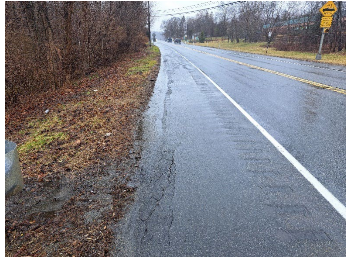
Photo 8-46: Storm run-off runs along the shoulder of Rt. 206 (Recommendation 20A)
